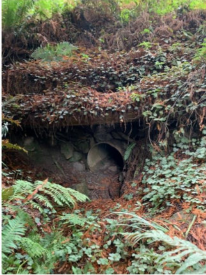
Railroad Ave #1 undersized failing culvert.
