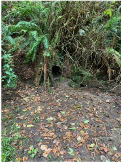
Railroad Ave #2 undersized failing culvert.
